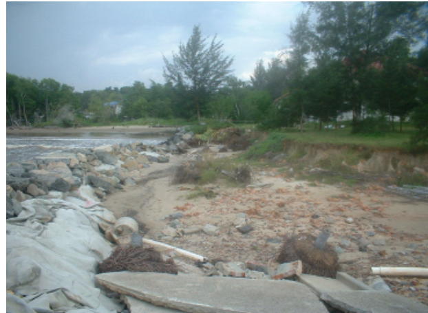
Figure 5: Failure of protection measure protection
